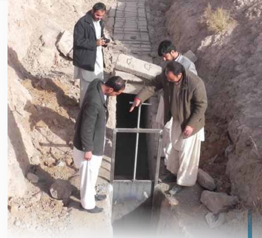
WATER MANAGEMENT: In a village in Afghanistan's Herat province, engineers and locals close down the karez for the winter. Built as part of the AWATT project, the newly lined and gated karezes enable farmers to manage the amount of water they can apply to their crops throughout the year.
