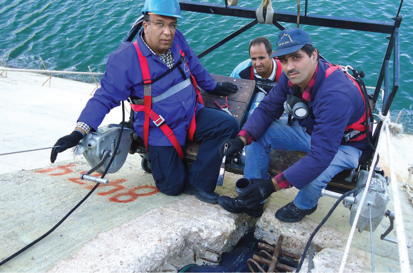
Technical staff members from the Litani River Authority rehabilitate the face joints of the Qaraoun Dam in Bekaa, Lebanon, through the USAID-funded Litani River Basin Management Support Program. The program inspected the dam in November 2010 to detect minor leaks from aged joints. | Photo: Nabil Amacha/Litani River Basin Management Support Program
