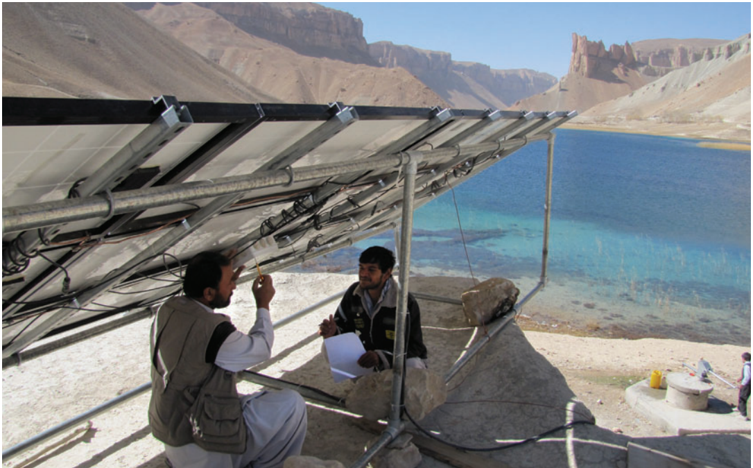
USAID is supporting the electrification of rural schools in Afghanistan through projects like the Afghanistan Clean Energy Program, which created a 2-kilowatt solar-powered system for Shaheed Mahmoodi High School in Band-e Amir National Park in Bamiyan Province. | Photo: Robert Foster/Winrock International
