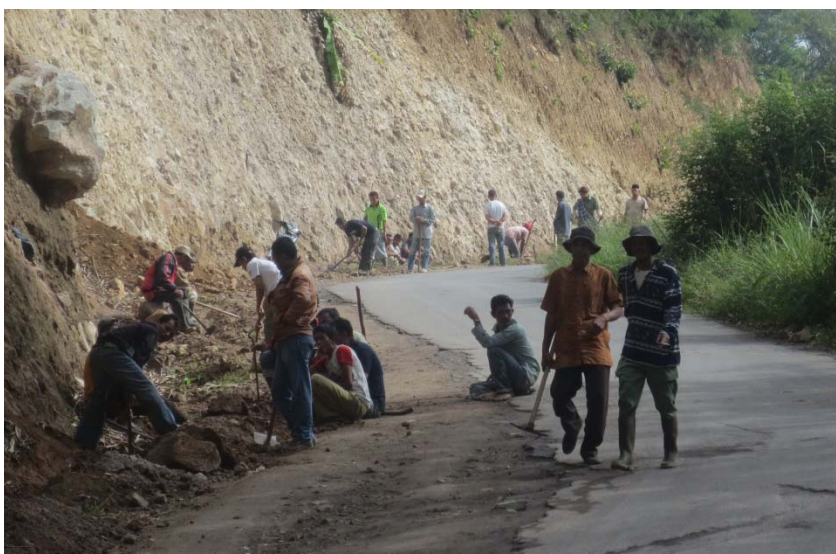
Workers dig a drainage ditch along a road in Aceh to help reduce flooding. (Photo by USAID/OFDA)
