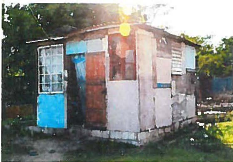
Houses built with unsafe materials and not up to code
