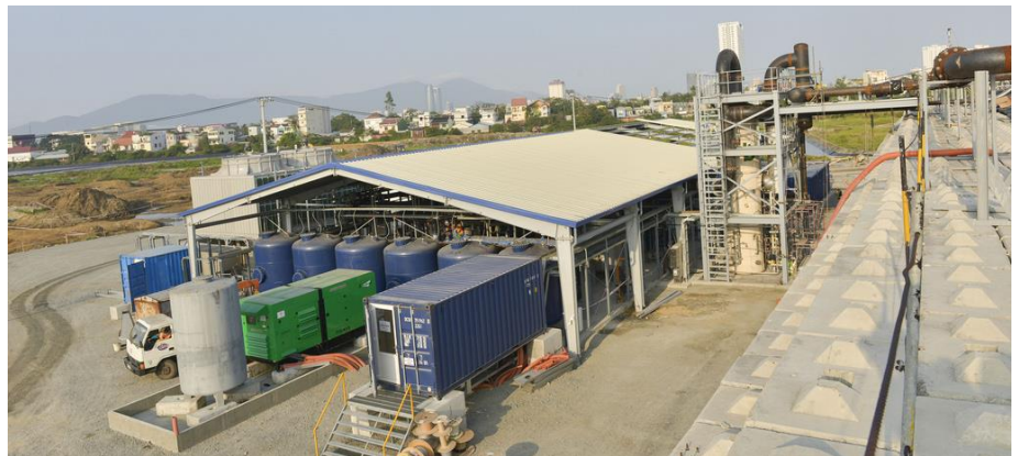
Liquid/vapor treatment plant at north end of containment structure
