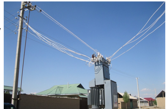
Several USAID programs support the Kyrgyz Republic's energy sector both in policy initiatives and infrastructure improvement. Photo: USAID
