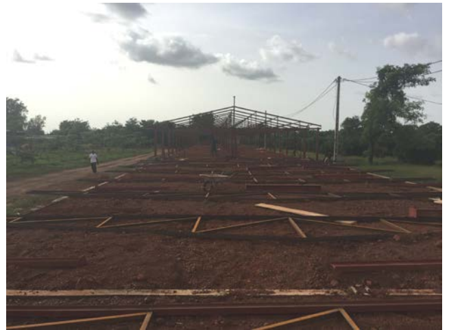
Farm shed in development for a project receiving support. Photo credit: MIFP
