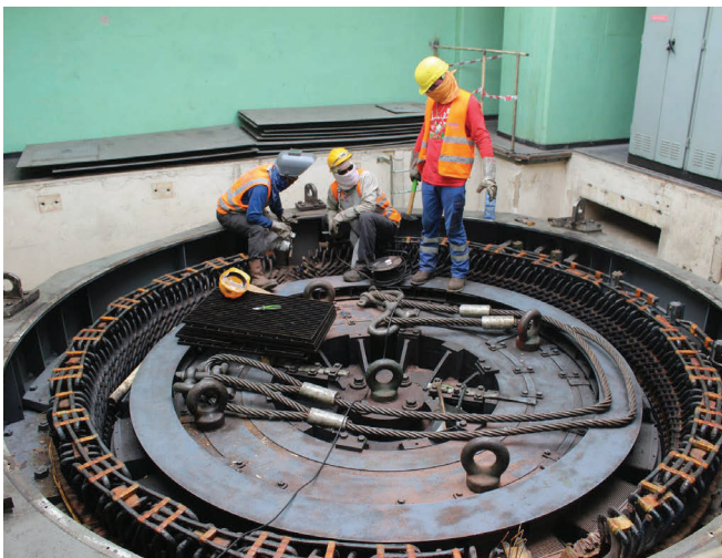
Nkula A Hydropower Plant in Malawi. Photo: MCC
