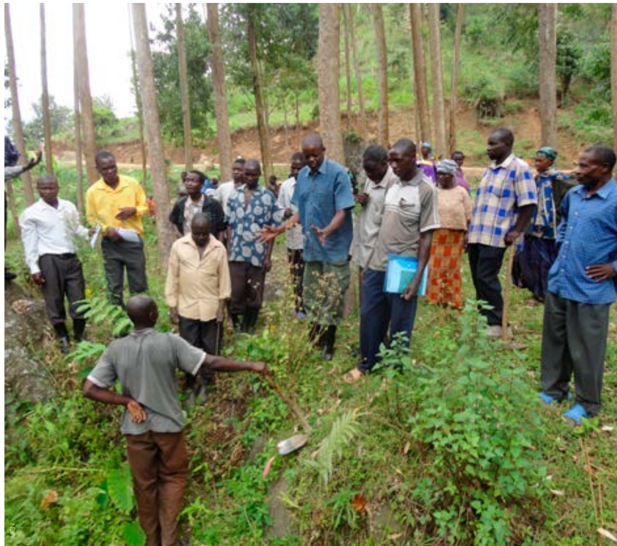
Photo above: Workers restore a river bank in the Manafwa Catchment of Mt. Elgon, Uganda.
